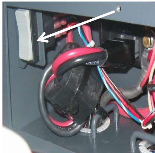
The switch is located behind the panel on the left side on the ER26.
